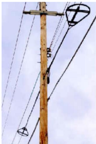
Figure 5 – Cable storage using snowshoes.
